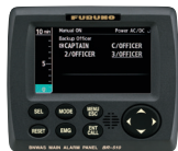
Main AlarM Panel
